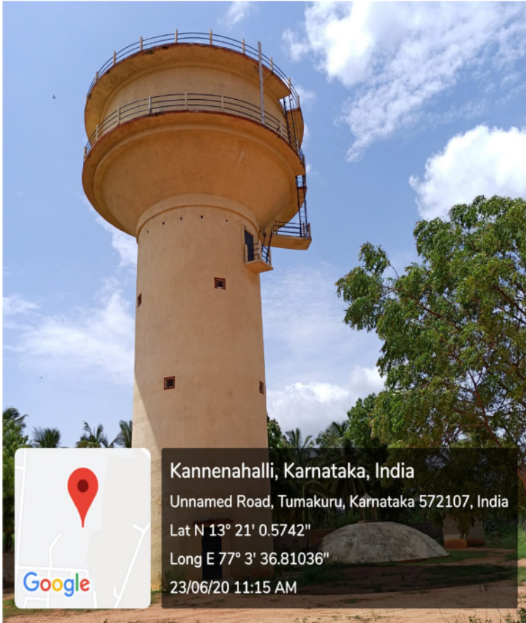
WATER STORAGE TANK
